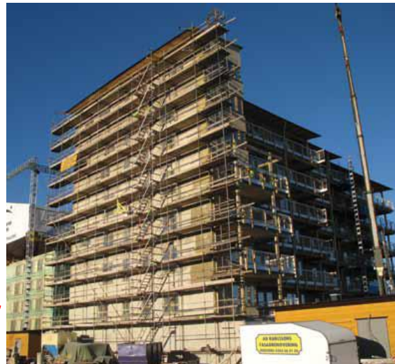
Växjö, Sweden/2008, Residential: 1+7 stories (last as duplex), 4 buildings, 10,700 m 2 CLT 4,800 m 3 , 4 days per floor
