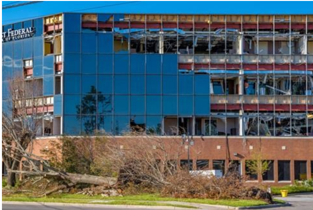
Slika 6 - Oštećenja zid zavesa usled dejstva jakih vetrova ( https://oceanimpactwindows.com/blog/window-breaks-during-hurricane/ )
