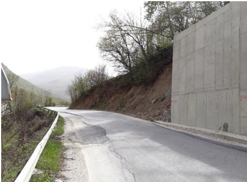
Figure 1 Landslide on the regional road Mavrovo-Debar
