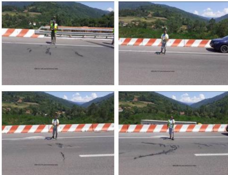
Figure 2 - Surface damage to the pavement [10]
