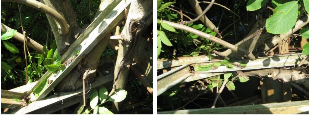
Figure 10 – Penetration of vegetation through the main beam of the bridge over Mlava river on the way to Rukumija monastery
