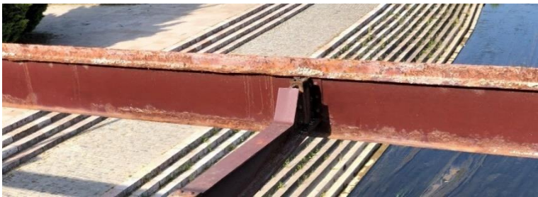
Figure 14 – General corrosion at the main beam of the bridge over Nišava river at the entrance at Nis Fortress
