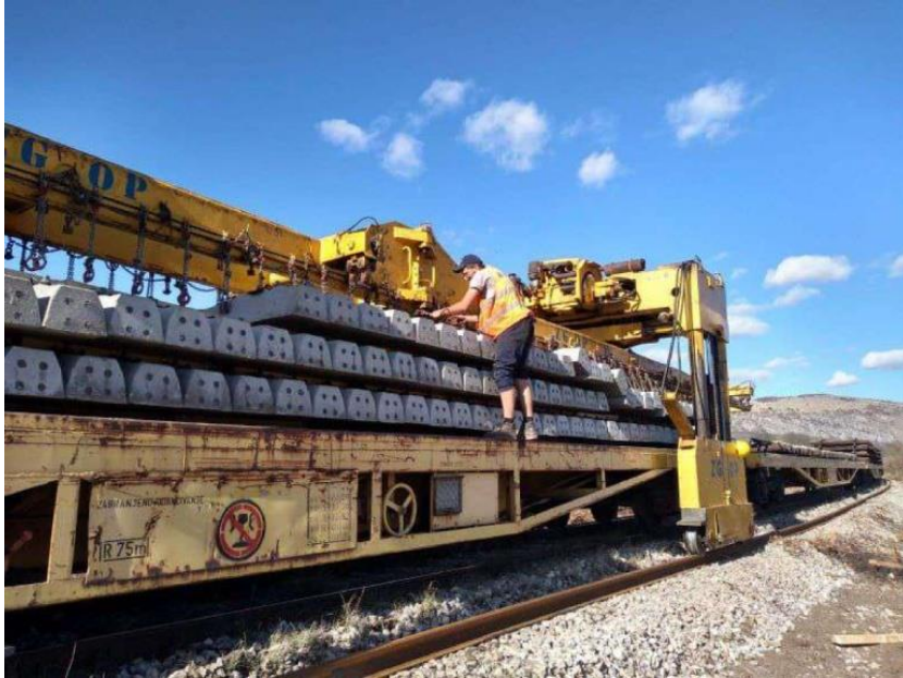
Figure 1. Removal of new sleepers from wagon plateau to intended position, using gantry crane (continuous method)
