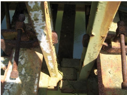
Figure 15 – Galvanic corrosion at parts of bridge over Mlava river in the way to Rukumija monastery
