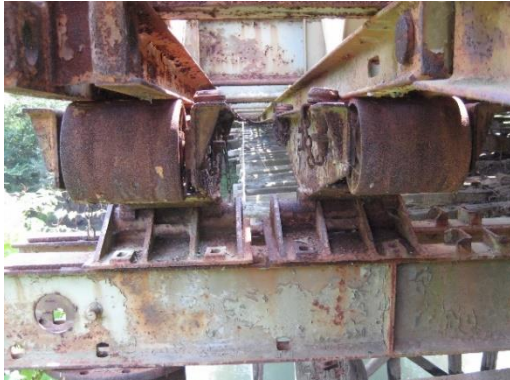
Figure 12 – Rust on supports of the bridge over Mlava river on the way to Rukumija monastery
