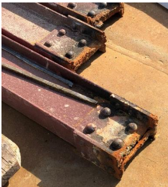
Figure 21 – Stress corrosion at transverse beams of the bridge over Nisava river in front of Nis Fortress
