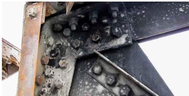
Figure 4 – The look of the connection of steel elements after fire
